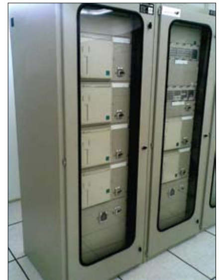
Fig. 2: The modern method of mounting the DPR in relay cabinets.
